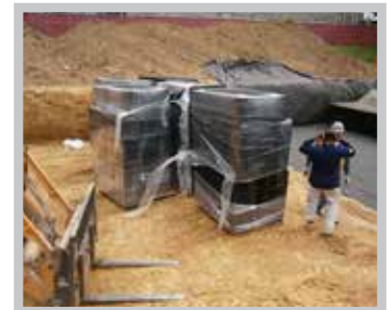
Figure 3 Installation can be sped up by either assembling the tanks in the excavation or placing the pre-assembled tanks in the excavation.
